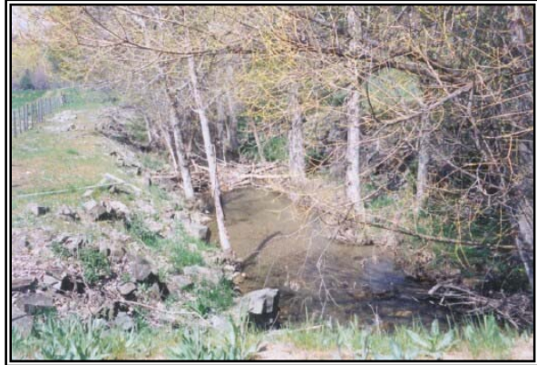
Photo 8. Portions of Moffett Creek has been channelized, riprapped. Willows planted during construction are now mature.
