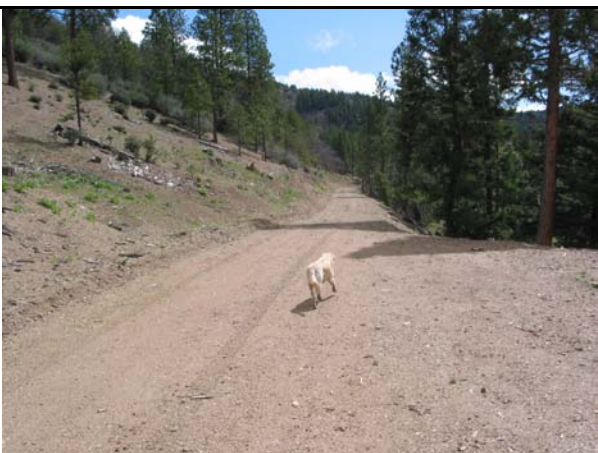
Photo 11. New road located and constructed to prevent erosion and to benefit stream/riparian recovery.
