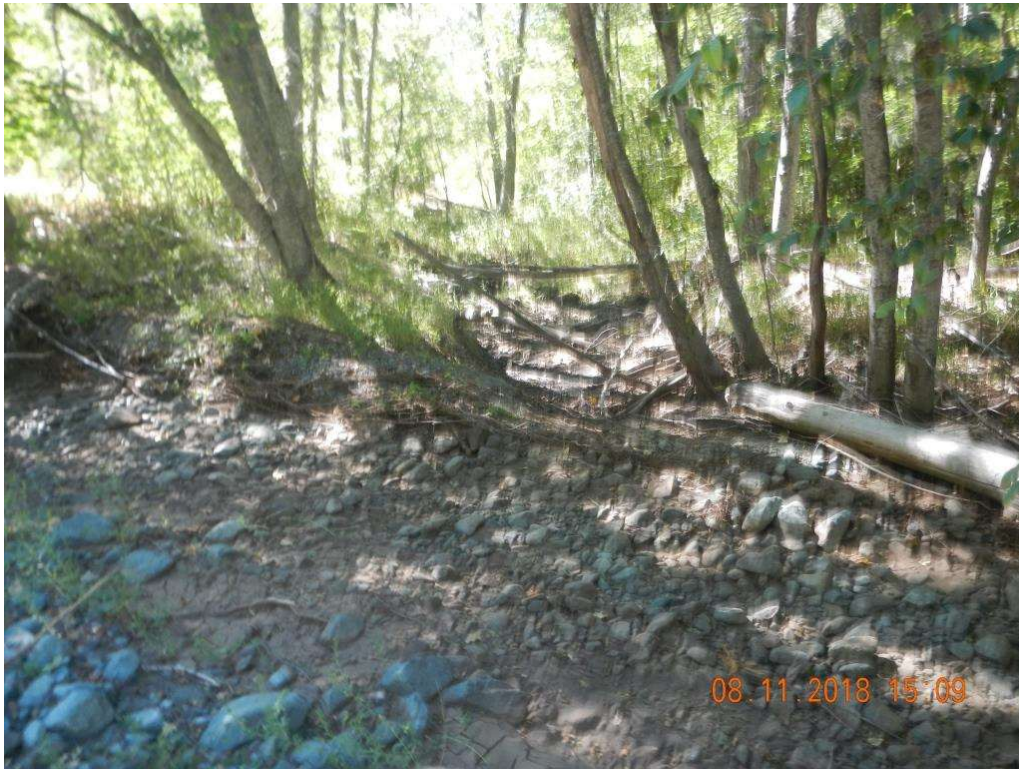
Picture 8 – Outlet of side channel (from Patterson Creek) in Phase II Reach
