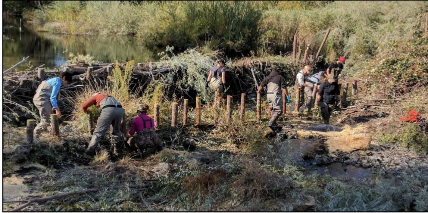
Figure 26. Construction of two step BDAs (BDA 1.1 and BDA 1.2) downstream of BDA 1.0 at Sugar Creek.
