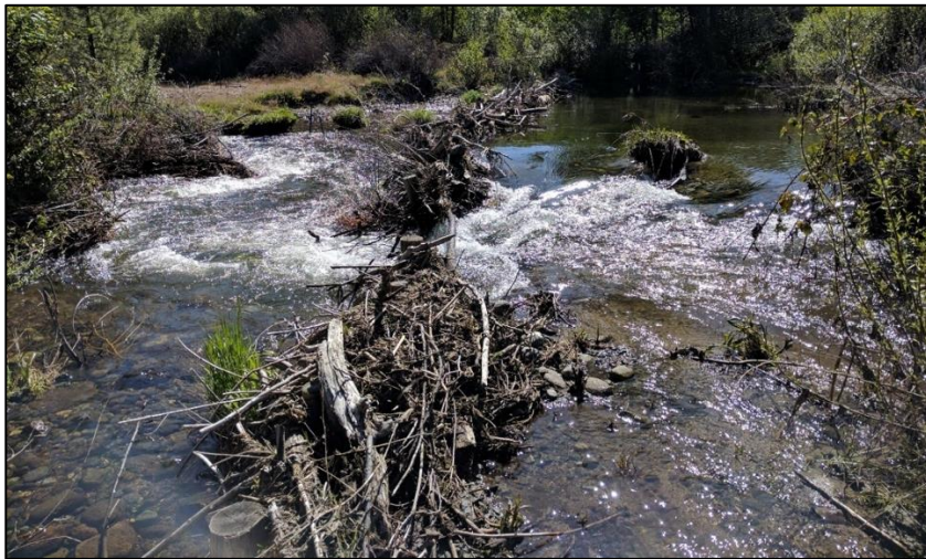
Figure 25. A 20-foot section of BDA 1.0 that was scoured during a February 2017 flood, resulting in the loss of four posts and associated weave.
