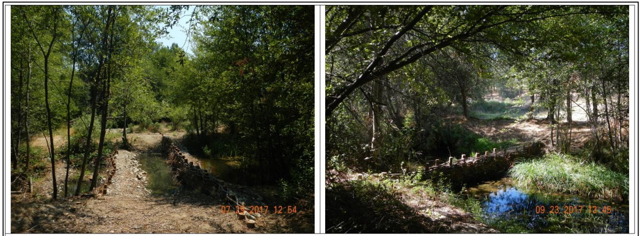
Figure 30. Feature photos. BDA 1 post construction. Photos taken from bank of mainstem French Creek, looking toward the side channel, now containing BDA structures.
