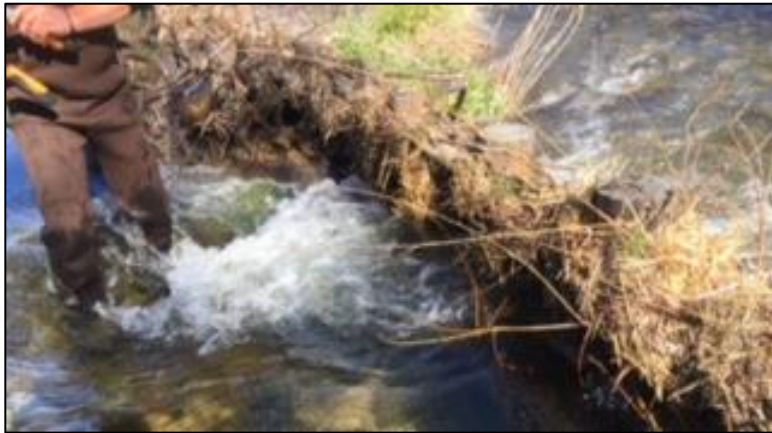
Figure 24. Scour hole undercuts BDA 1.0 at Sugar Creek.
