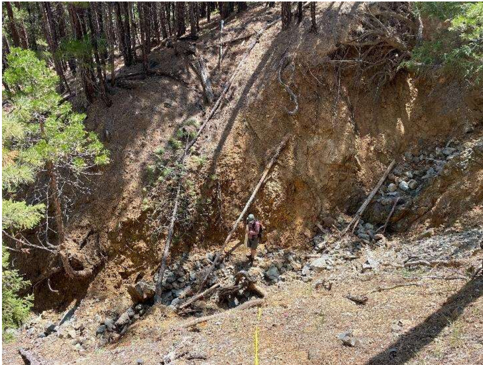
Photo 2.24: Maximum cross-section in Gully Complex 8 is 800 ft 2 . EFG8f. May 29, 2023.
