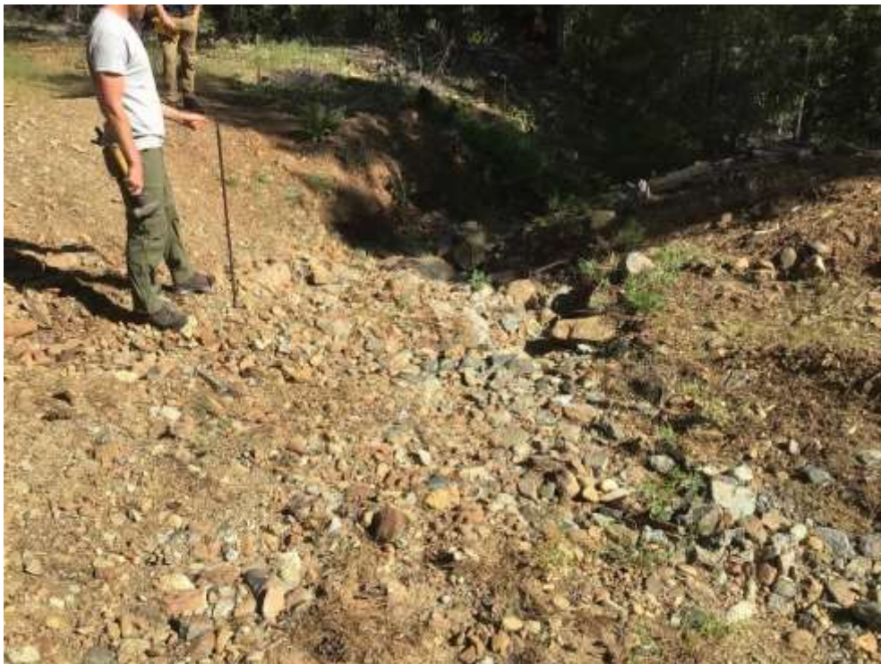
Photo 2.48: Gully Complex 5 road crossing. EFR6. May 23, 2023.
