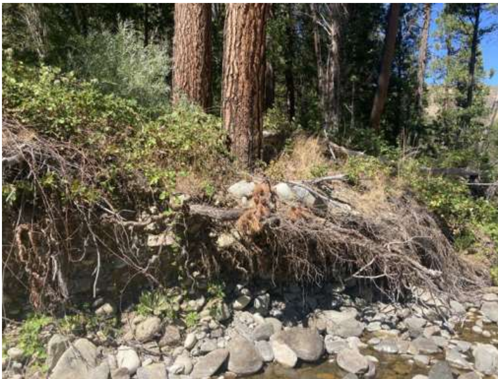
Undercut roots of ponderosa pine at RKM 5 cutbank
