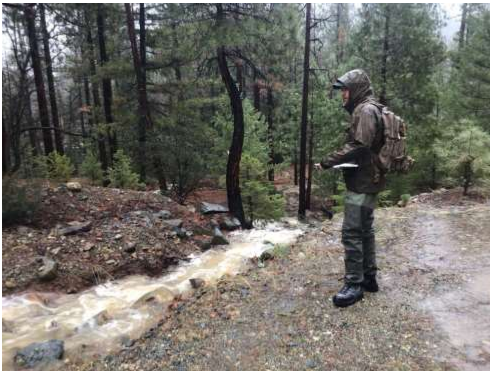
Photo 2.6: Erosion of road fill. EFR2. January 13, 2023.
