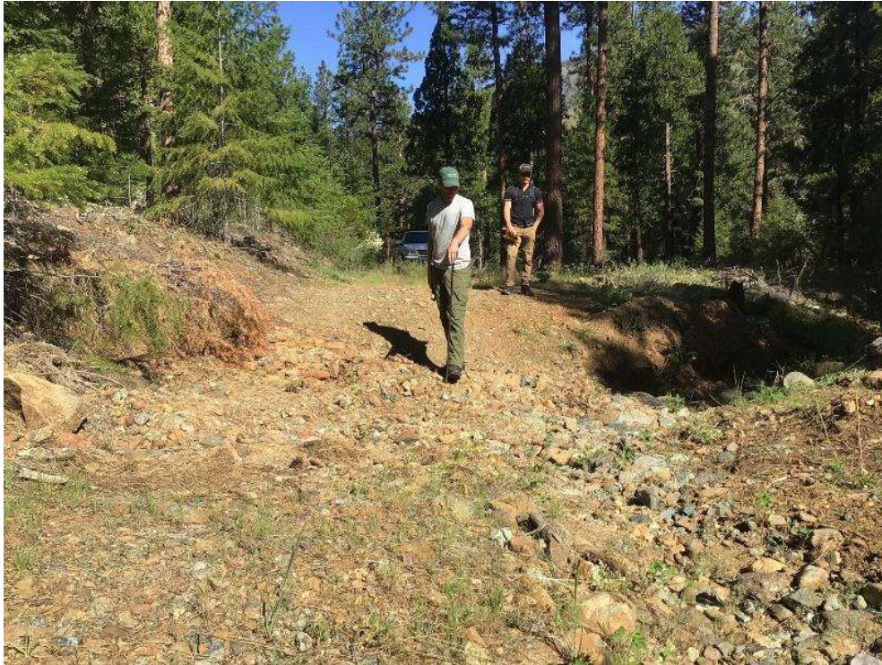
Photo 2.47: Gully Complex 5 road crossing. EFR6. May 23, 2023.
