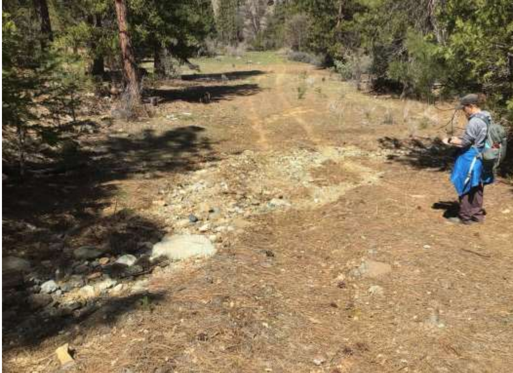
Photo 2.3: Example of extreme erosion point, EFR13.1; April 13, 2023.
